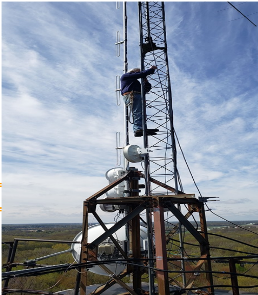
When climbing Ron found feed-line from another antenna was wrapped up in our antenna.
